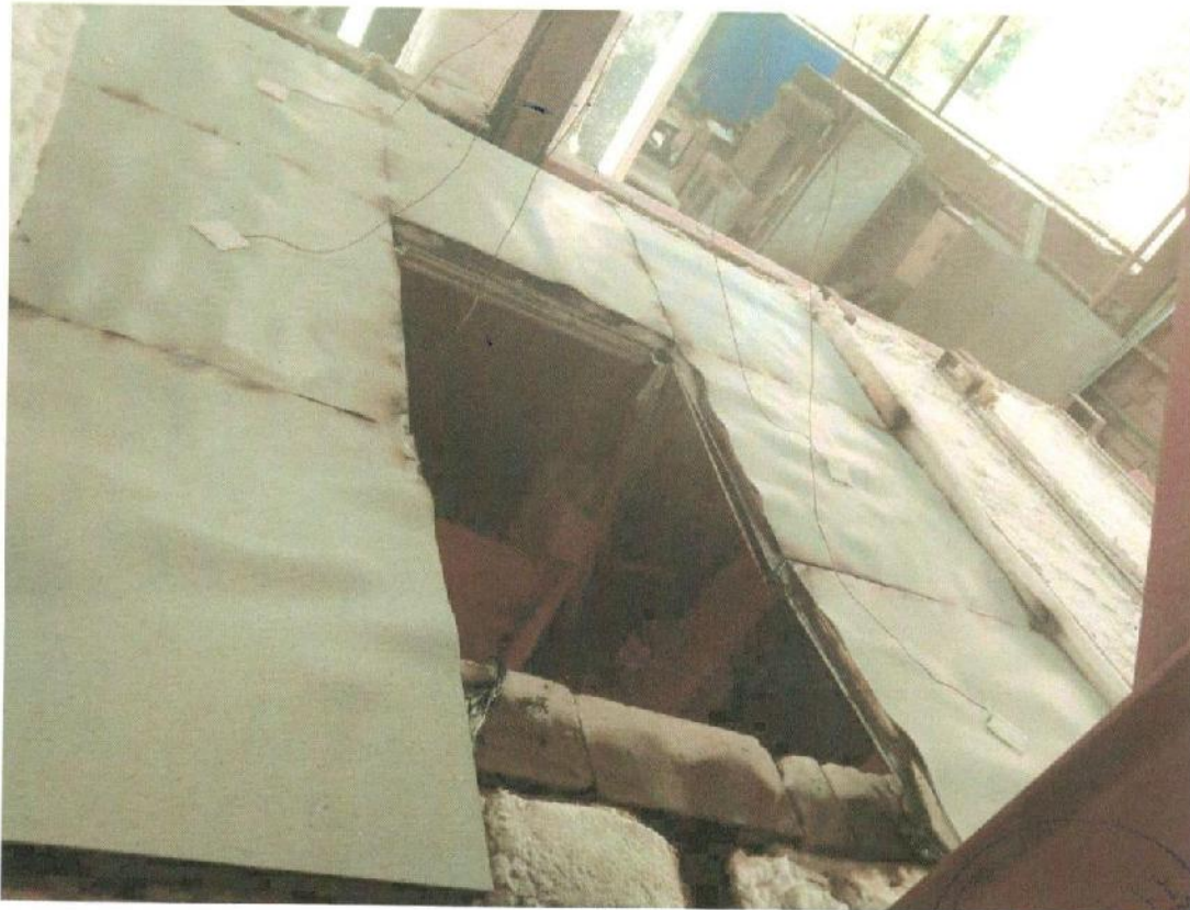
Figure (4): the tested sample after the fire resistance test.
